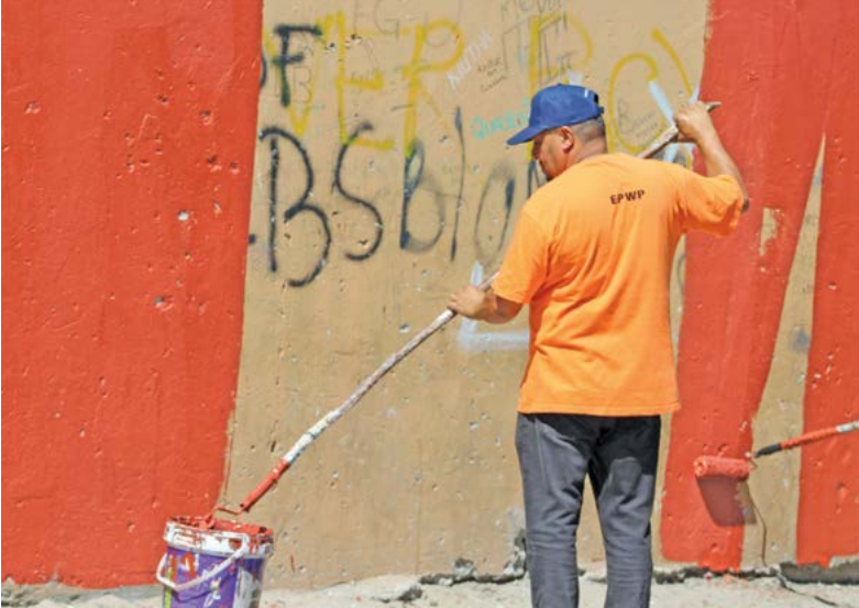
Got it covered: In the last three months of 2025, the City's Graffiti Unit removed nearly 10 000 m² of illegal graffiti.
